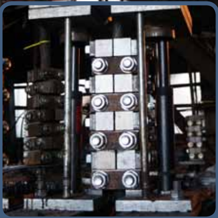
Each of the 14 wire ropes, which weigh 14 tonnes each including weights, is fitted with eight 2-bolt clamps and then raised using a hydraulic jack sufficiently to allow a second set of clamps to be installed below the first.
