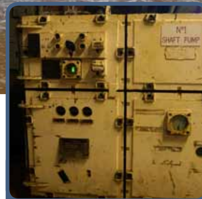
The maintenance aspect of the contract aims to ensure continued efficient operation of the pumping and treatment equipment
