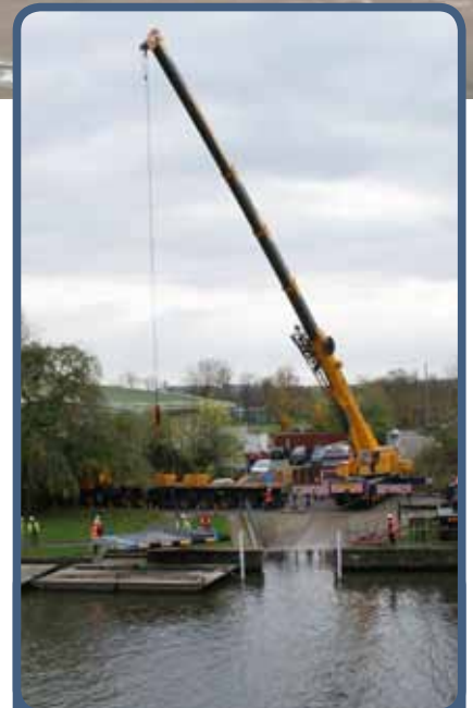
The new lock gates will be designed by ECS, according to the specifications provided by the EA
