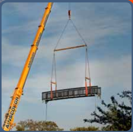
The new maintenance-free bridge was designed and manufactured by ECS from recycled plastic and a steel sub-frame.
